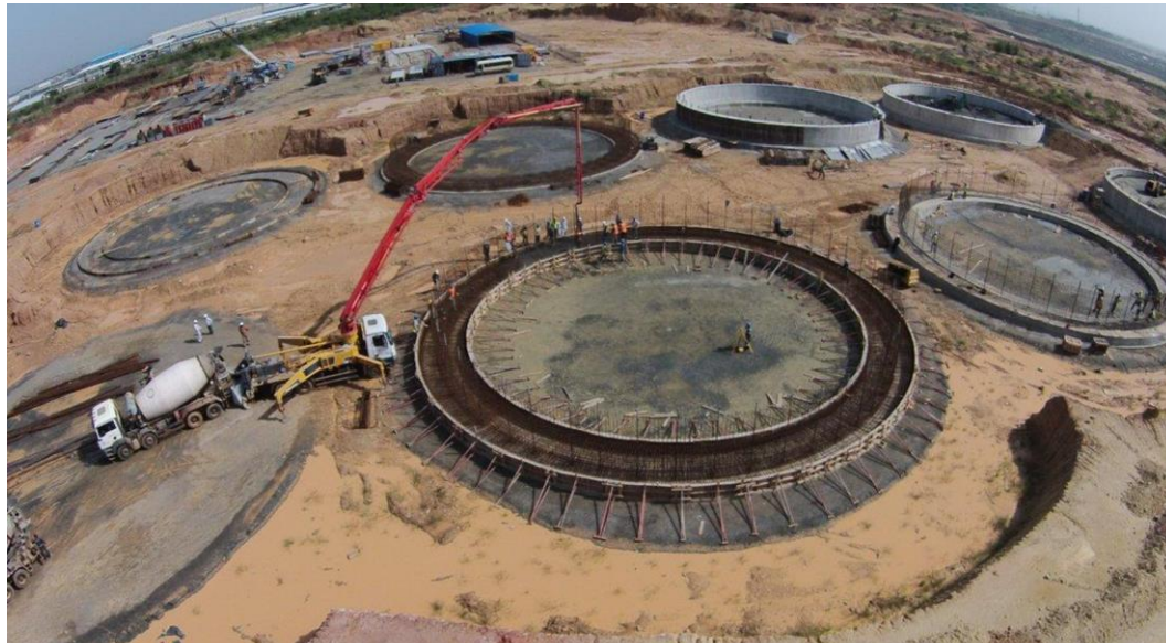
Example // PUMA ENERGY Terminal (Ghana)
